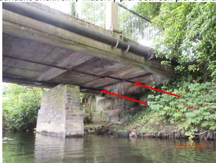
Picture 25 - metal service pipes suspended beneath bridge deck
